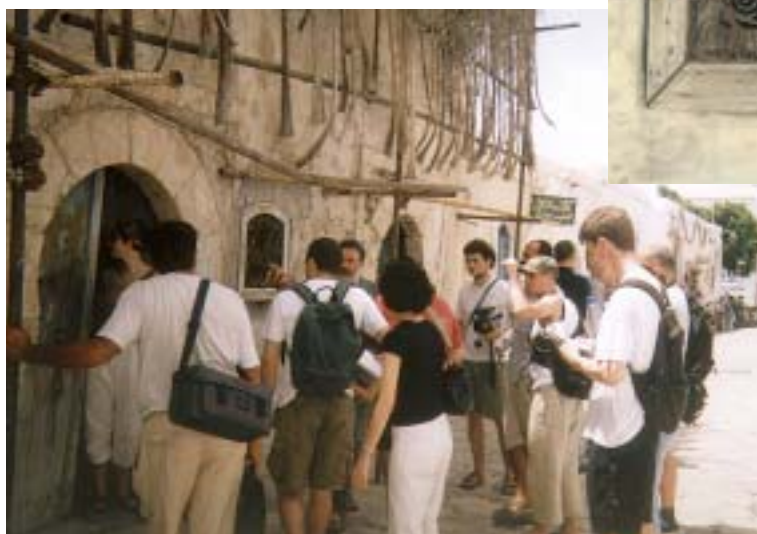
Tunisian and French students examine the restoration work of the façade of a demonstration house in Mahdia, July 2002. Above right: Detail of the demonstration house.
