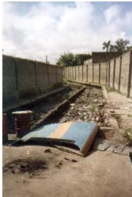
Debris and garbage blocking a drainage channel in Ikoyi Island, Lagos, Nigeria, July 2002.
